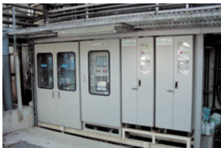
Wastewater continuous monitoring device
