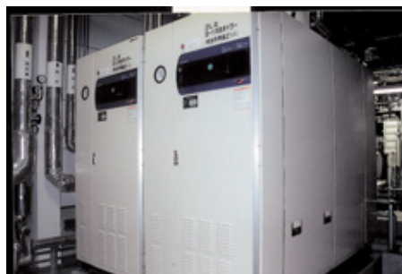
Natural gas boiler
