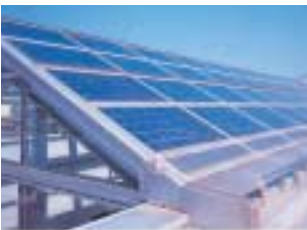
ROHM Fukuoka solar energy generation facility Annual power generation capacity of 22,000 kwh
