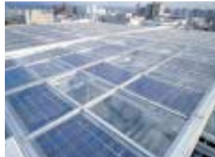
ROHM head office solar energy generation facility Annual power generation capacity of 11,000 kwh
