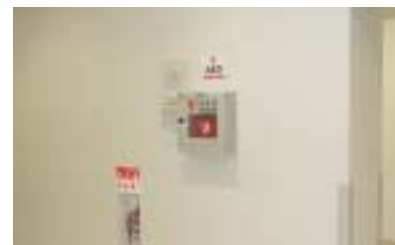
An installed AED
