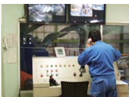
Central Management Room for Production Process
